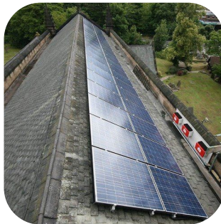
Solar Photovoltaics at St Mary's, Moseley
